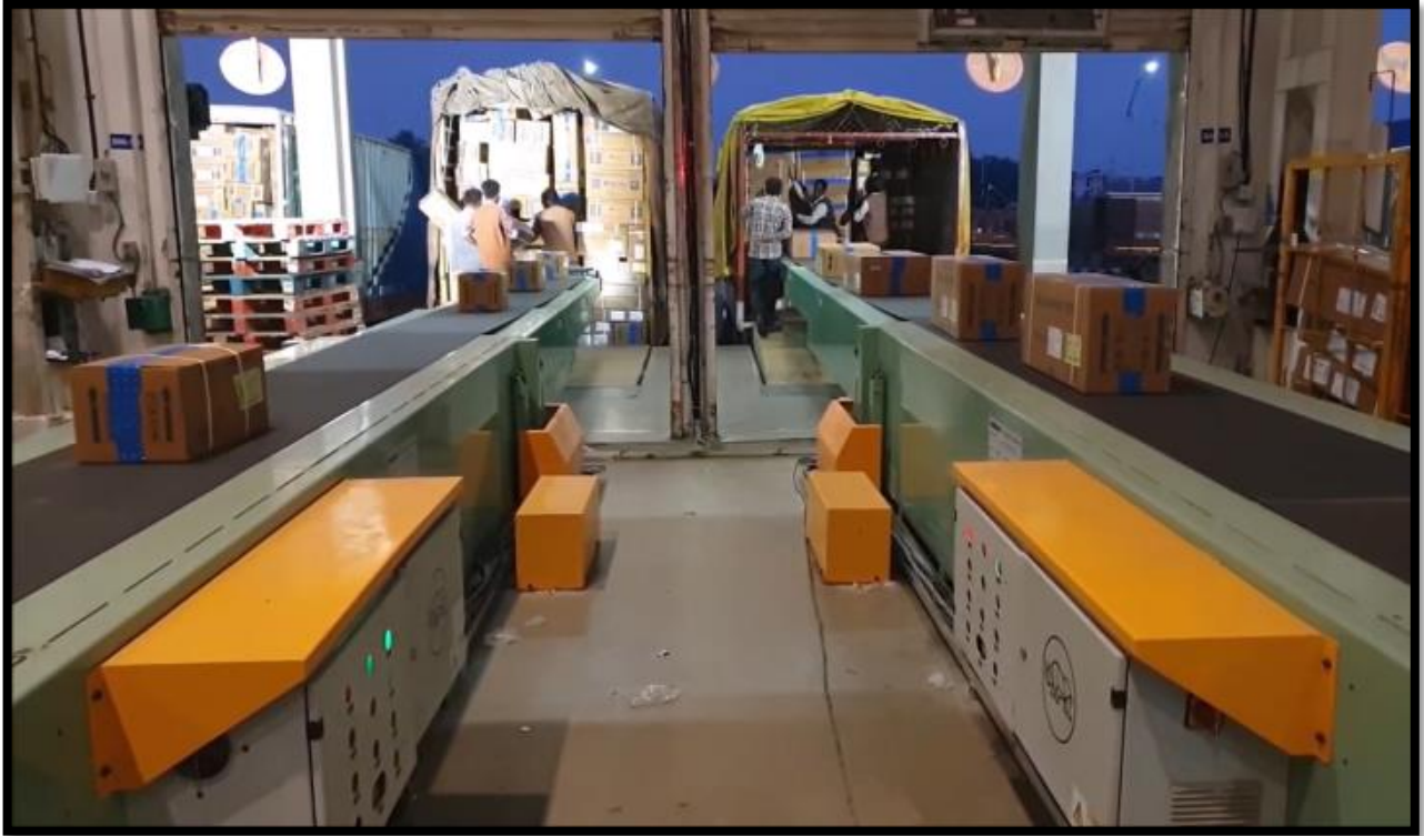
NIDO Verification System in two outbound docks
