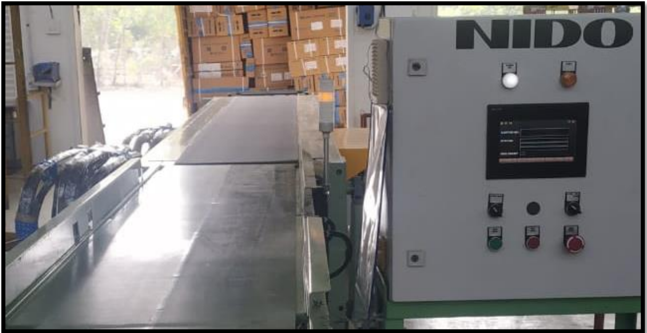
NIDO Verification Conveyor with Control Panel
