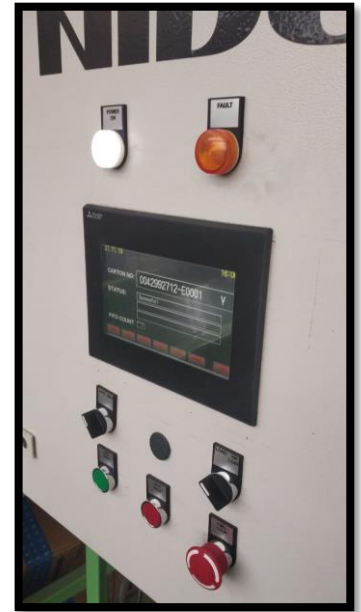
HMI Control Panel
